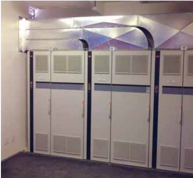
These VLT® AutomationDrive frequency converters with back channel cooling control motors in the mine dewatering system. They are installed in the MCC substation.
