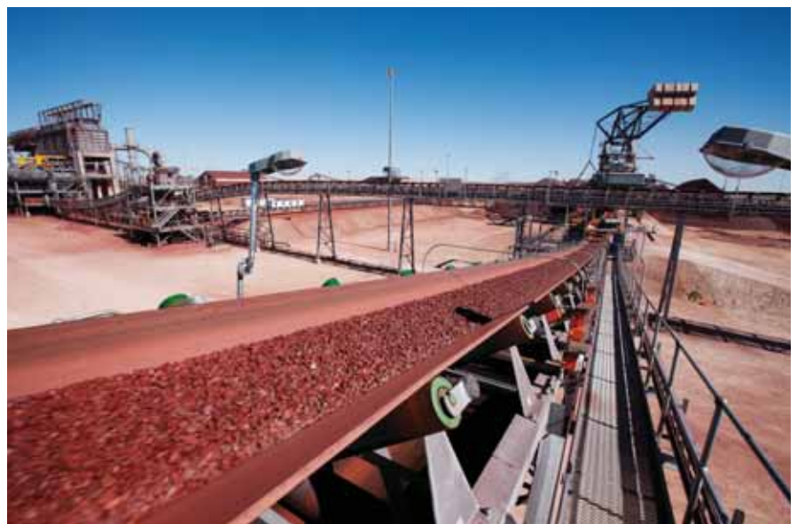
Graded iron ore being transported by conveyor to the load-out terminal at Kolomela
