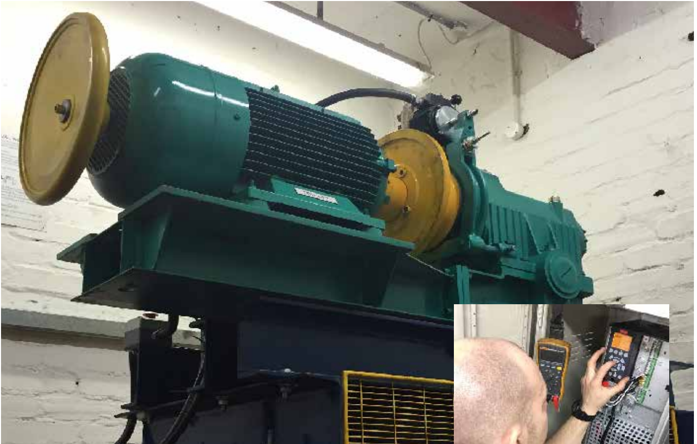
The drive for the elevator motor had failed and needed replacement.
