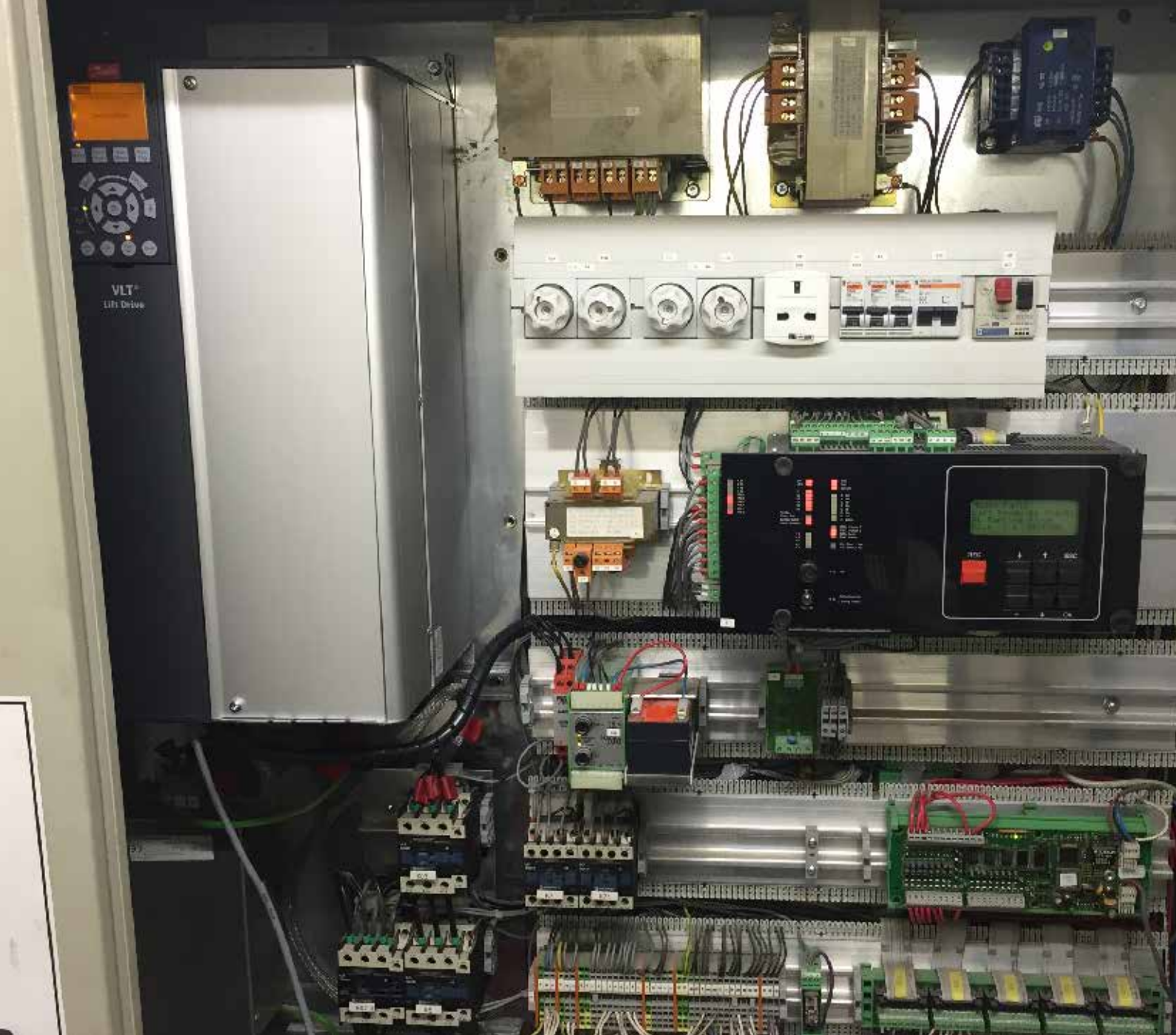
Installing the Danfoss VLT® Lift Drive was straightforward due to designed-for-the-job elevator functionalities.
