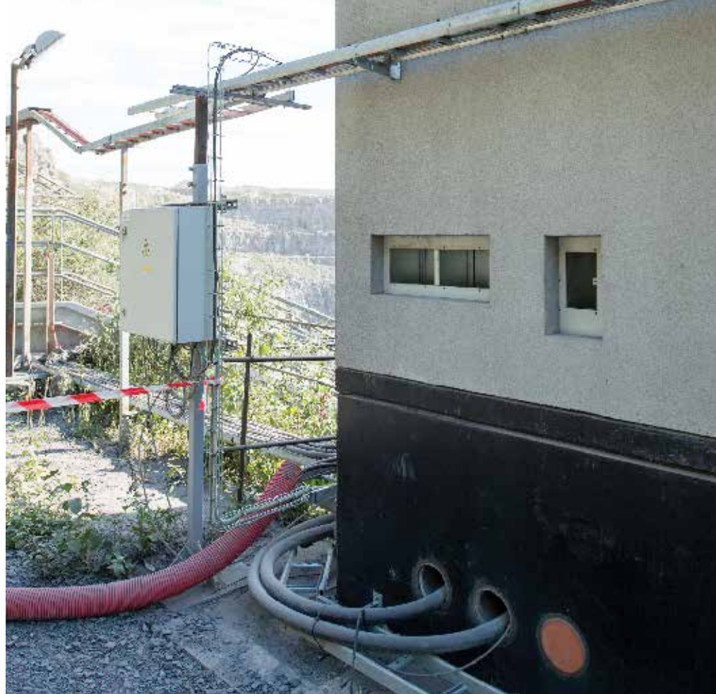
90% of the heat generated by the AC drive bypasses the technical room.
