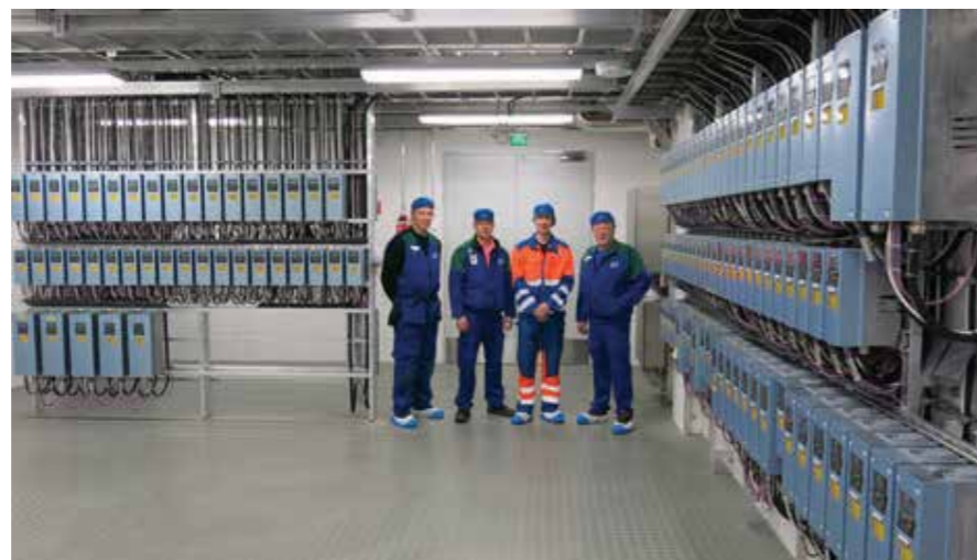
All VACON® AC drives delivered to the Seinäjoki plant are provided in splash-proof IP54 enclosures. Hannu Teräväinen (front left), Pauli Parvi, Teemu Takala (back left) and Marko Vähäkoski inspecting one of the electrical rooms.
