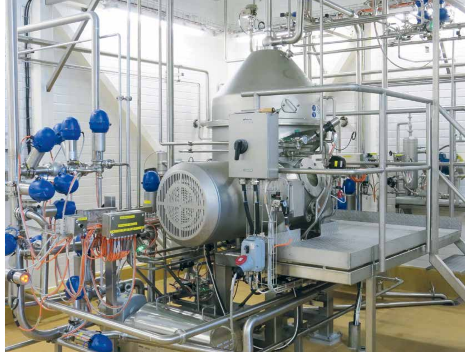
Valio's Seinäjoki plant produces all Valio quarks. A separator is used for producing quark. The pumps and mixers used by the separator are controlled by VACON® 100 AC drives. In recent years, quarks have been the quickest-growing product category in retail sales. Valio was able to quickly double its production at the Seinäjoki plant as butter production had recently moved to new premises.
