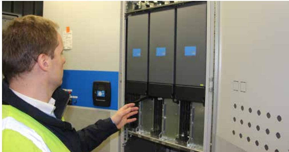
Sverre Knapstad, Frekvensomformer.no demonstrates the VACON® NXP modules installed inside the container
