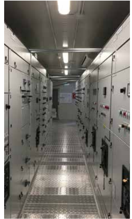
Inside view of a container made by Casagrande Elettrocostruzioni for the Edinburgh Energy from Waste plant
