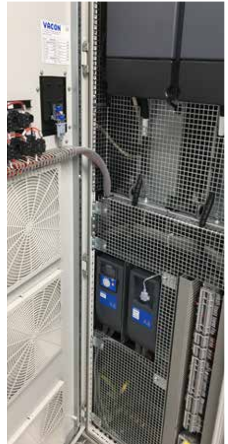
Detail of the electrical panel made by Casagrande Elettrocostruzioni housing Danfoss Drives VACON® NXP
