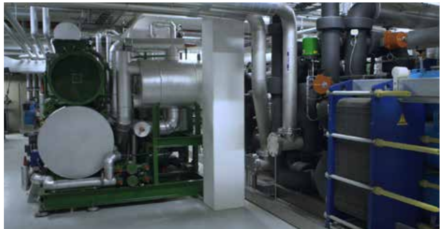
The cooled water from the heat exchanger is circulated in the building to cool rooms to the desired temperature. No active refrigeration is required.
