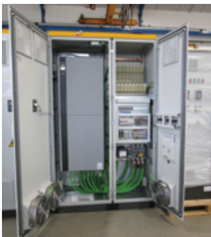
Electric control panel -FC102
