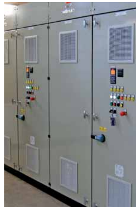
Motor control panels at Affinity Water
