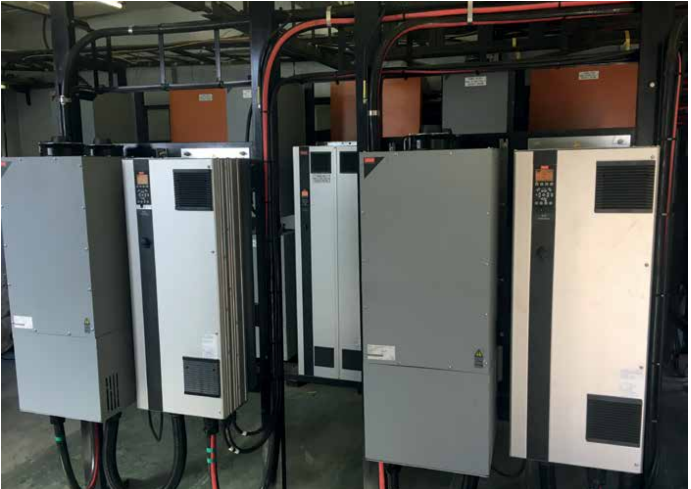
The process cooling water (PCW) system now benefits from VLT® AQUA Drive controlling each of three cooling water pumps, and VLT® HVAC Drive controlling both the cooling tower fans.
