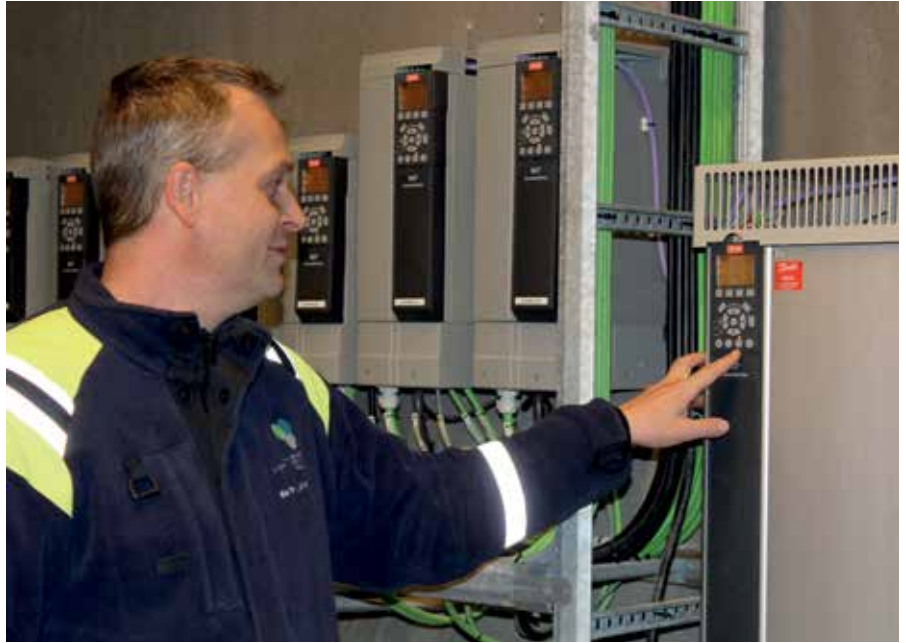
Martin Lorentzen, Electrician, next to a 45 kW VLT® AutomationDrive FC 302 drive.
