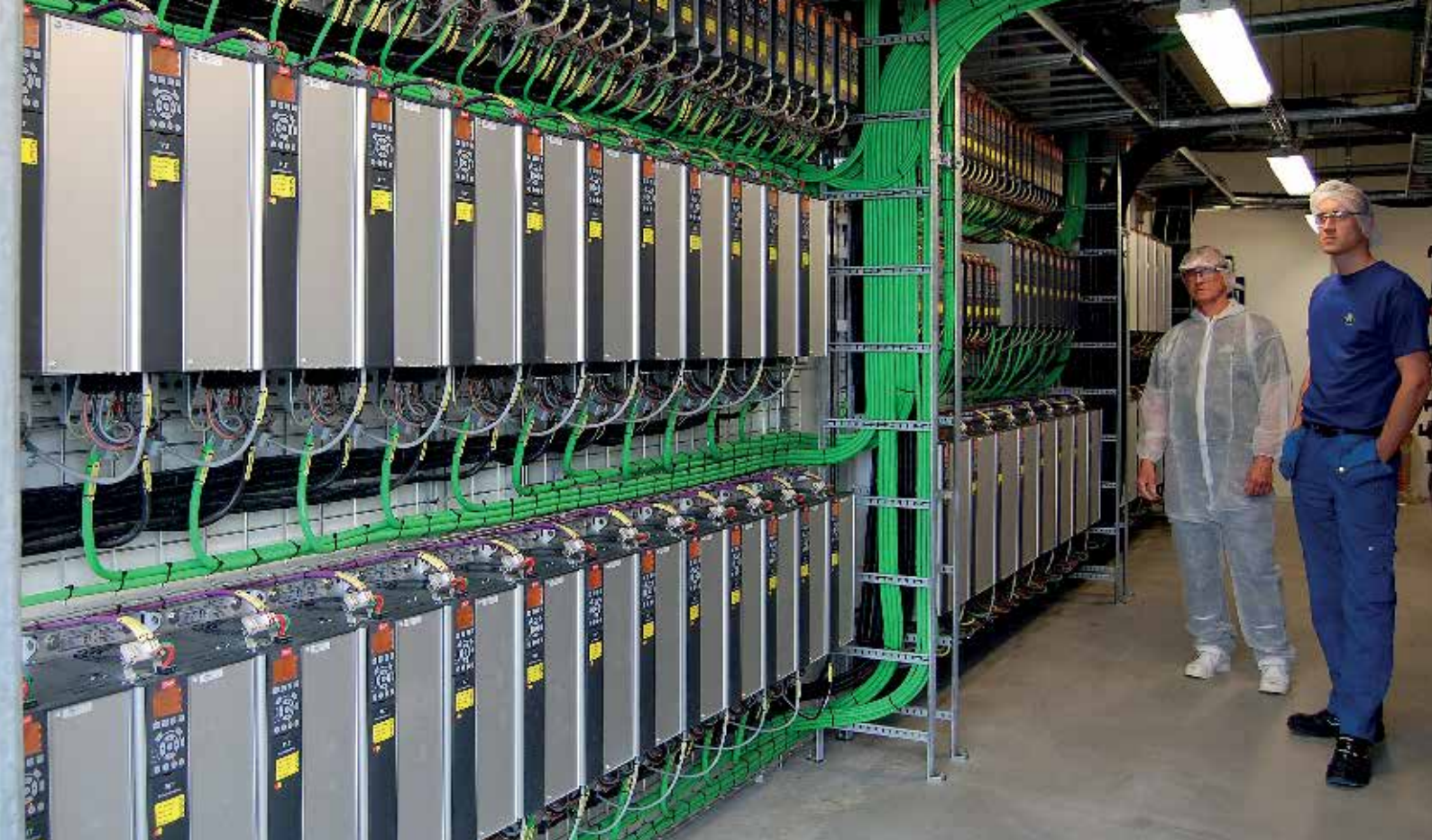
The 1400 VLT® drives are mounted in a series of well-ventilated control rooms, with no need for cabinets. From left Knud Rahbek and maintenance manager Simon Arentoft
