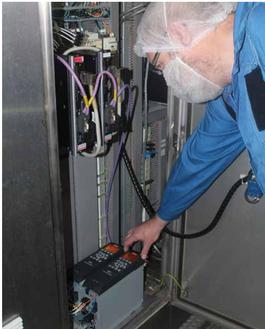
The VLT® AutomationDrive with Integrated Motion Controller provides significant cost and time savings at Danish Crown.
