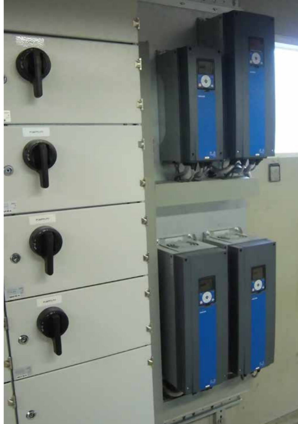
VACON® 100 FLOW units at the Osvald waste water pumping station. The drives were installed on a backplate at SK-kojeisto, the Seinäjoki, Finland based company that has built the switchboards used at KRS-Vesi.
