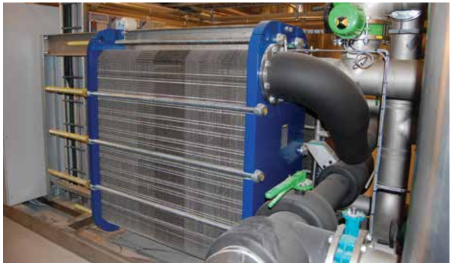
The cooled water from the heat exchanger is circulated in the building to cool rooms to the desired temperature. No active refrigeration is required.
