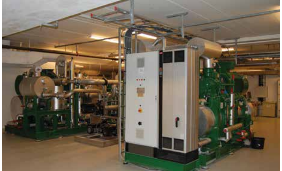
Two AC drives in the form of 355 kW VLT® HVAC Drive FC 102 IP54 control the screw compressors which enable the two GEA Greenco heat pumps with a combined performance of 2,400 kW to adjust the heat capacity continuously from low to full performance, with the same efficiency.
