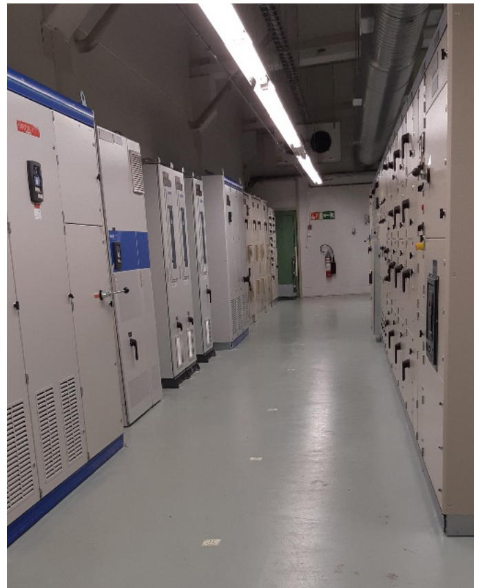
VACON® drives in the pulp mill's control room Image: Metsä Fibre Oy
