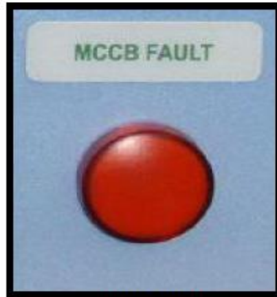
Figure 7-5. MCCB FAULT indicator
