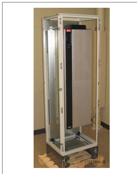
Illustration 3.36: Frekvensomformer installeret i kabinettet
