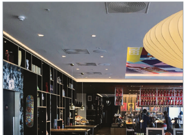
The SEM-SAFE® high-pressure water mist nozzles fits perfectly with the modern interior of CitizenM Shoreditch Hotel.
