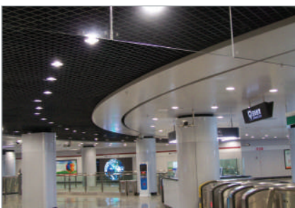
Access area to the metro protected with SEM-SAFE®.
