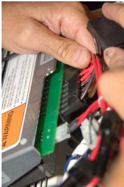
Figure 5 Connect Test Harness to Soft-Start Board (As Seen From Top Side of Board)
