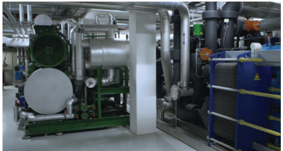
The cooled water from the heat exchanger is circulated in the building to cool rooms to the desired temperature. No active refrigeration is required.
