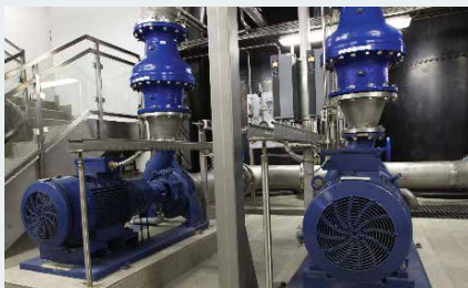
Water supply, Wertheim, Germany Raw water from deep wells is treated in a three stage process. VLT® AQUA Drives make it possible to balance these three processes to maximise treatment performance.
