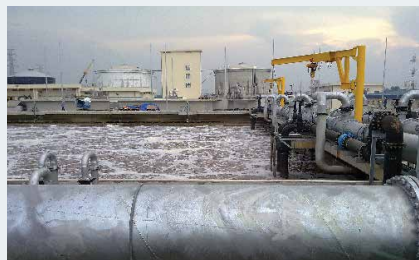
Wastewater treatment, Hanoi, Vietnam The wastewater treatment plant, Yen So Park, treats 50% of Hanoi's wastewater. More than 90 VSDs are installed, of which 12 450 kW VLT® AQUA Drives control the blowers.
