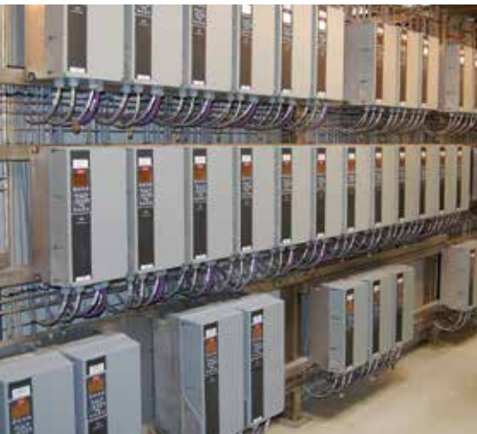
A typical drive installation with multiple frequency converters all installed on the same power supply often requires supplementary harmonic mitigation to avoid harmonic voltage distortion.
