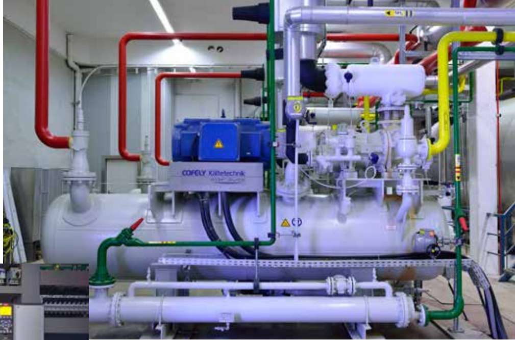
Three screw compressors with a refrigerating capacity of 2,700 kW guarantee the required level of cooling, whereby a 315 kW Danfoss VLT® HVAC Drive frequency-controlled compressor drive supplies the base load.
