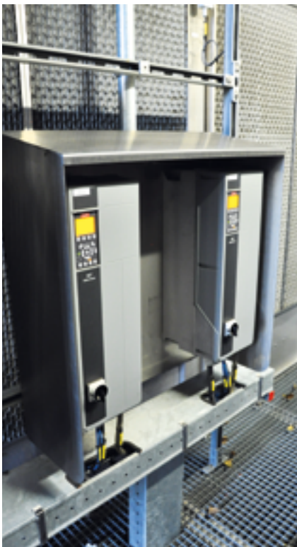
Outdoor installation for the regulation of the cooling towers, comprises two VLT® HVAC Drive FC 102 drives in IP55 enclosures, with built-in disconnect switch.
