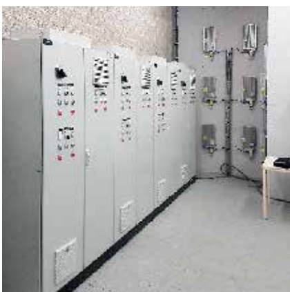
One of the two technical rooms with brake resistors at the end wall.
