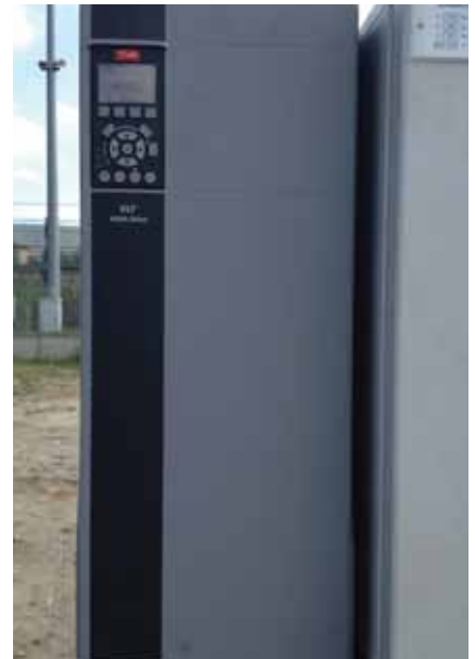
VLT® AQUA Drive FC 202 IP66 frequency converter installed outdoors, adjacent to the water collection tank
