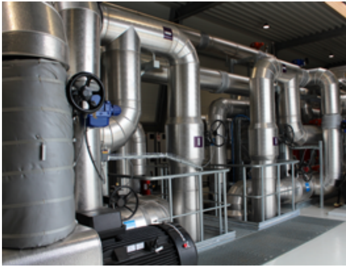
VLT® AQUA Drive FC 202 controls all eight pumps at Silkeborg water heating plant.
