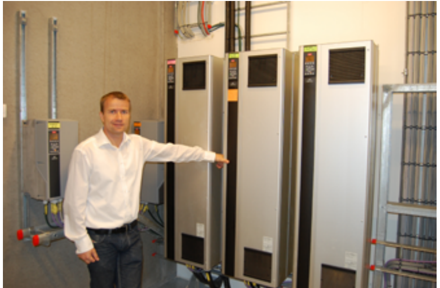
Jan Dong Høgh, District Cooling Manager at Copenhagen Energy in front of VLT® High Power Drives.
