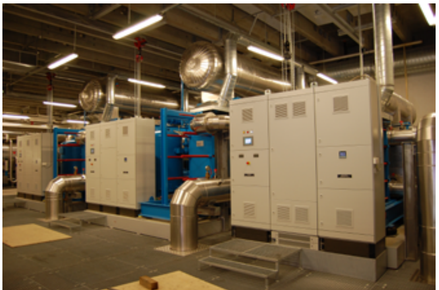
The refrigeration system comprises two 3.5MW screw compressors and one 1.3MW reciprocating compressor.
