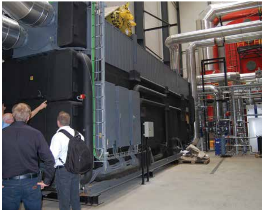
Absorber in the foreground. Scrubbers in the background.
