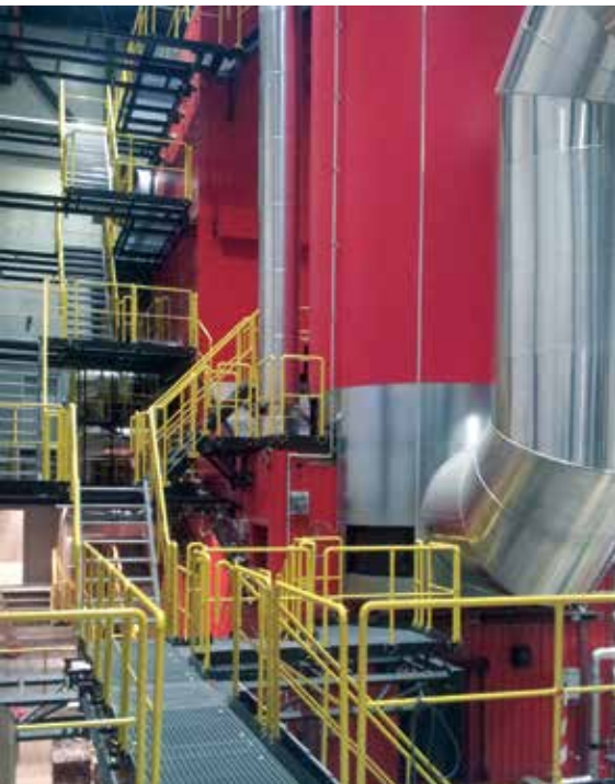
Vertical biofuel boiler and flue gas shotblast cleaning.
