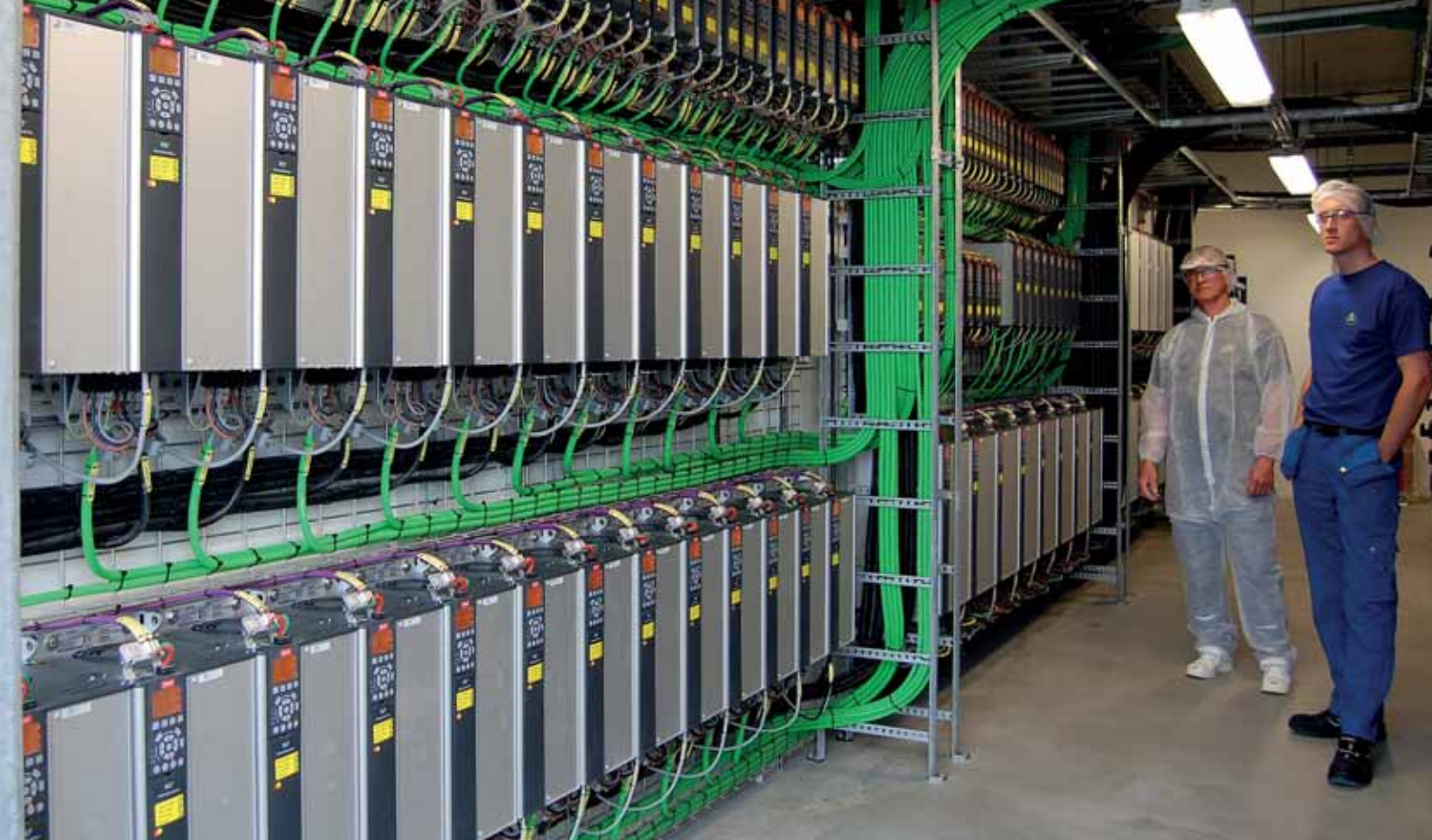
The 1400 VLT® frequency converters are mounted in a series of well-ventilated control rooms, with no need for cabinets. From left Knud Rahbek and maintenance manager Simon Arentoft
