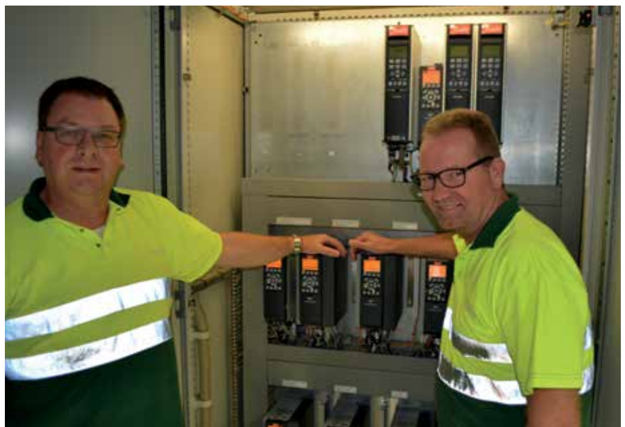
Control unit with VLT® AutomationDrive FC 302 drives, with Jan Brouwers, detail engineer, and Berry de Vaan, detail engineer software, at Heineken in 's-Hertogenbosch.
