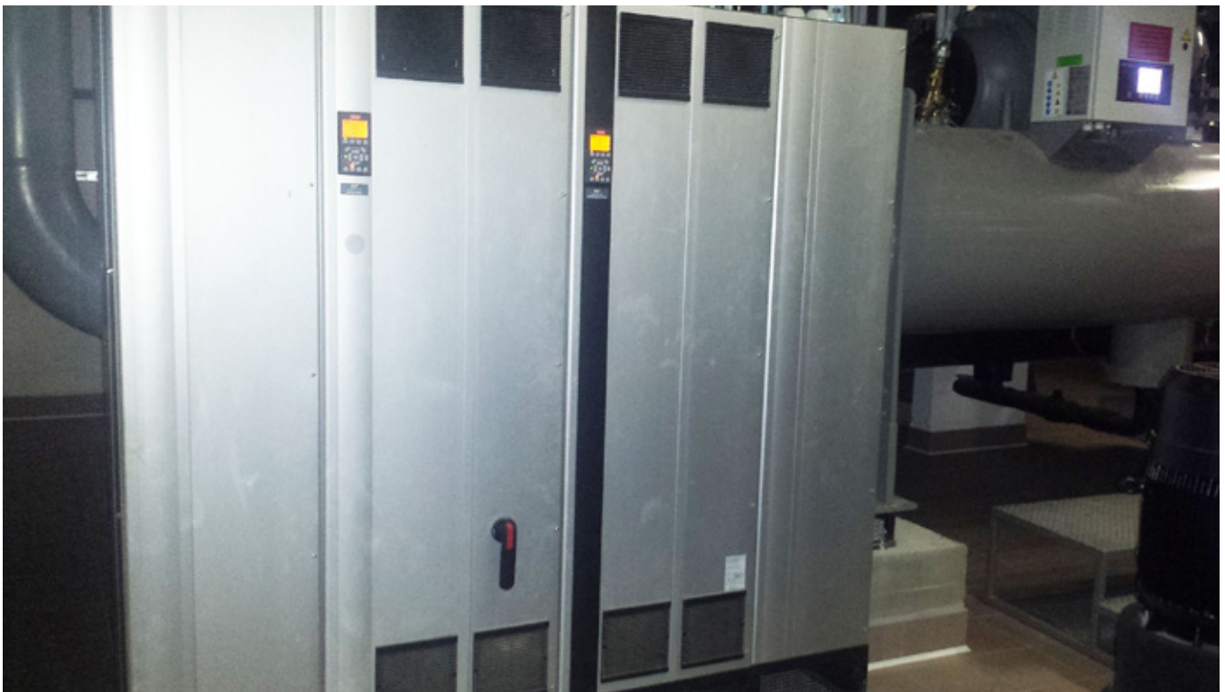
These VLT® Low Harmonic Drives control the new compressors in the machine room.
