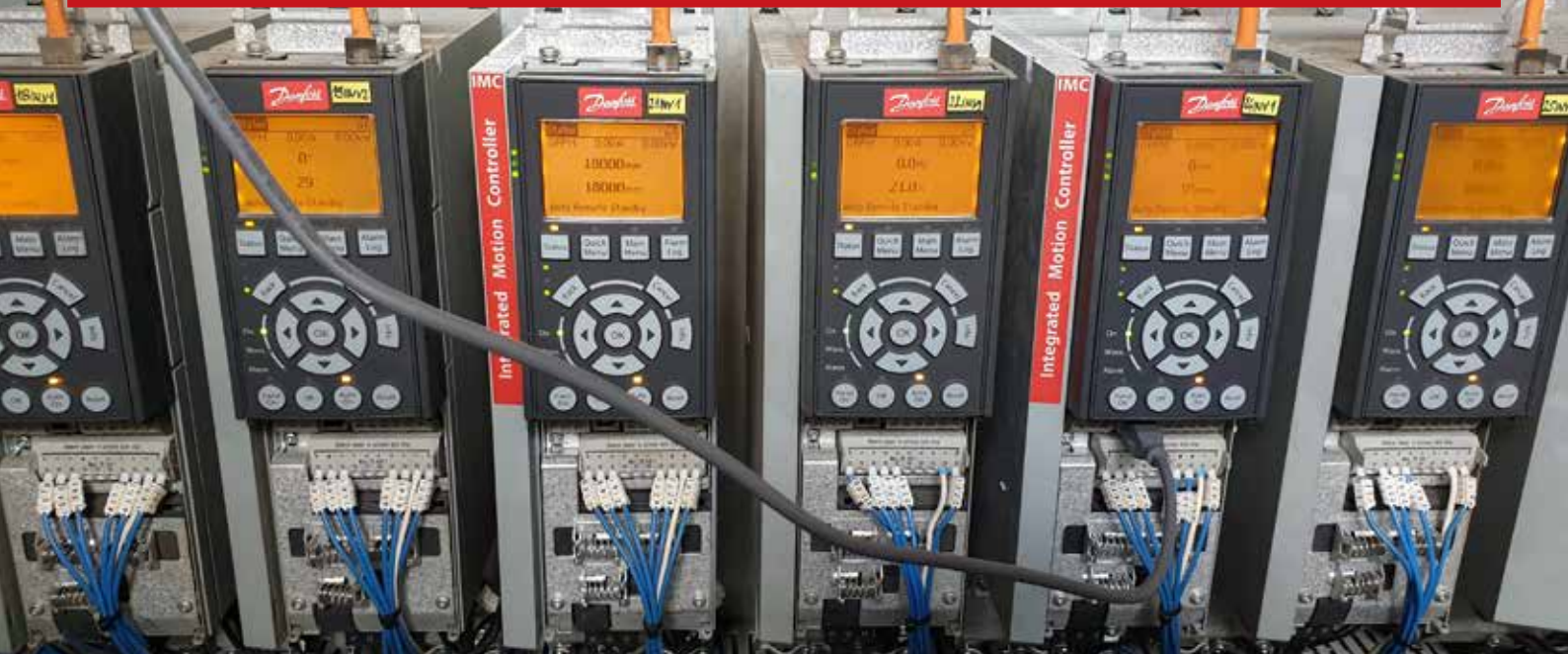
Blue cables show comms from encoder - yellow cables are for Modbus TCP comms
