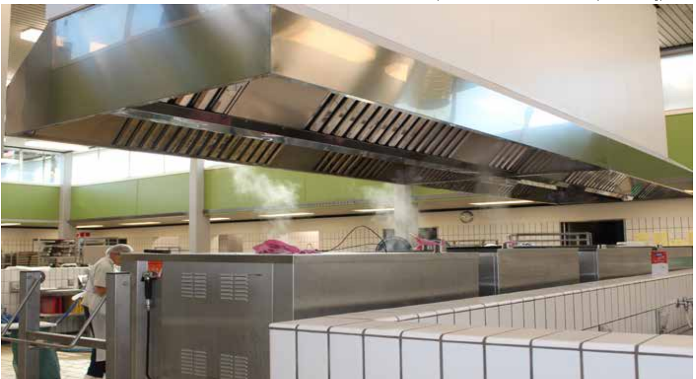
The new ventilation system includes a renovation of the ventilation room for the industrial kitchen, as well as a new ventilation system for the basement and nearby dermatology clinic
