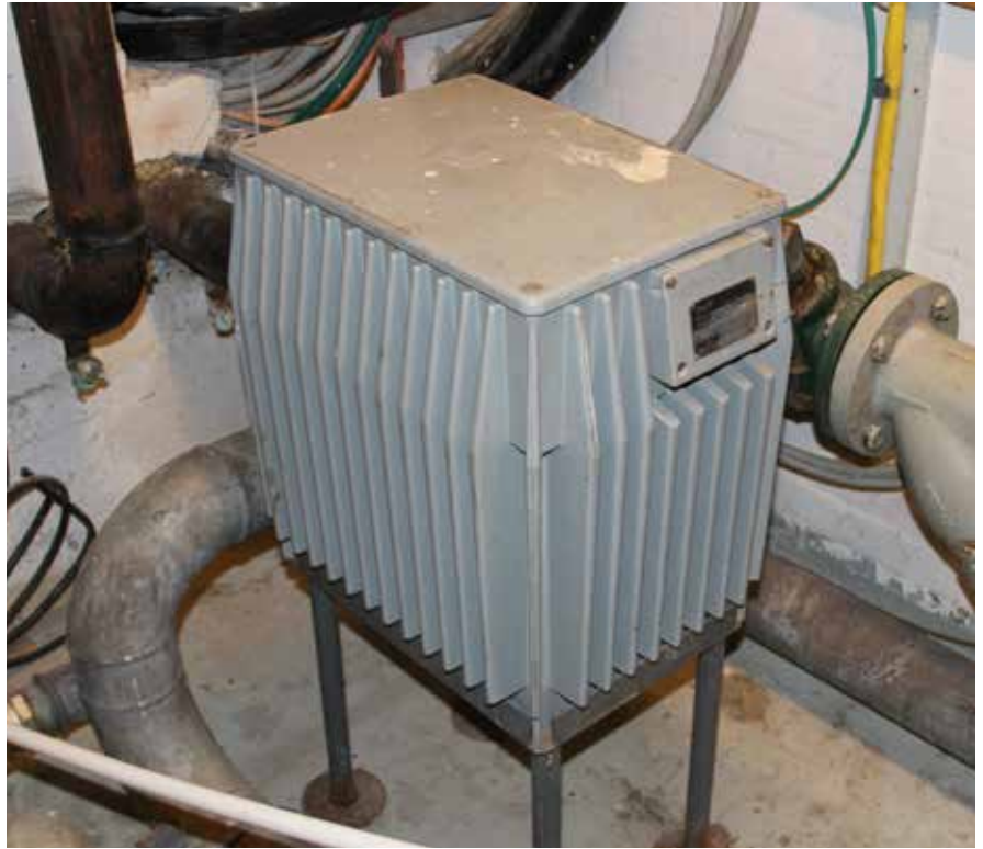
This VLT® 5 drive has ensured reliable, low-energy ventilation for Tønder Kommune in Denmark for more than 40 years
