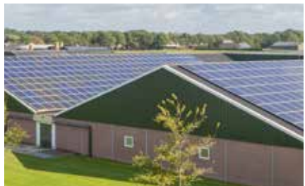
▲ Roof-mounted solar panels
