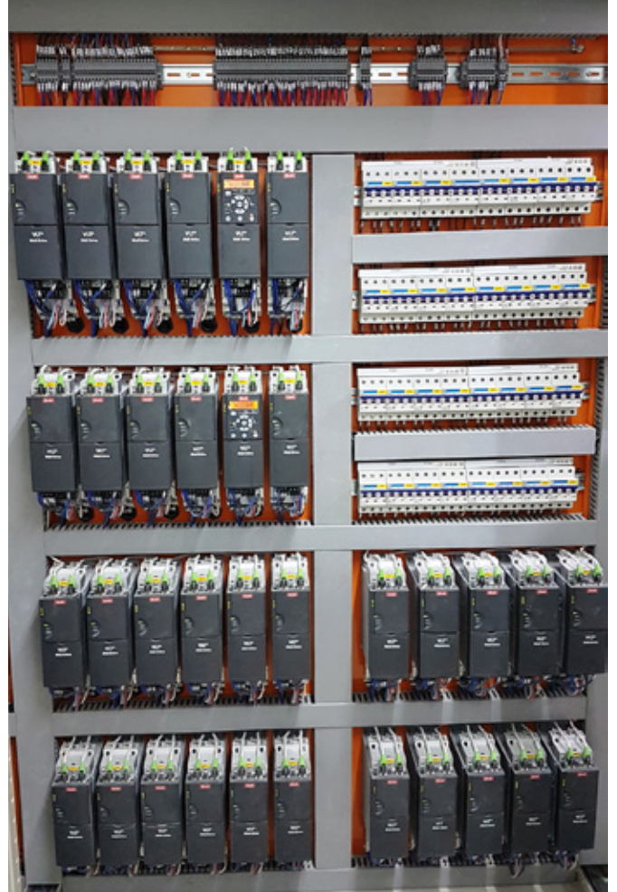
In total, the biscuit factory boasts 100 installed VLT® Midi Drives, controlling equipment as varied as fans, conveyors and mixers.
