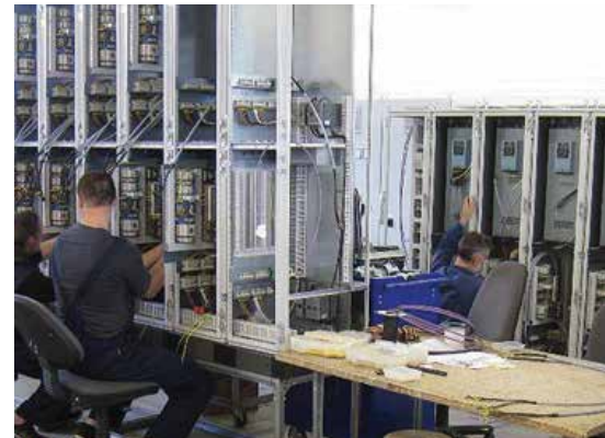
VACON® Active Front-End/common DC bus units being installed in switchgear. Vacon's Active Front-End technology complies with the most stringent harmonic distortion requirements, set by the Norwegian classification body Det Norske Veritas. If required, it also enables the energy generated by winch braking to be fed back into the vessel's electrical network.
