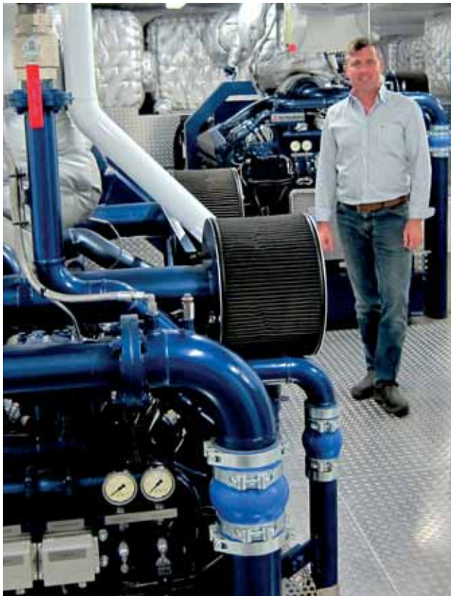
One of the main diesel engines (foreground) and the generator set (background).
