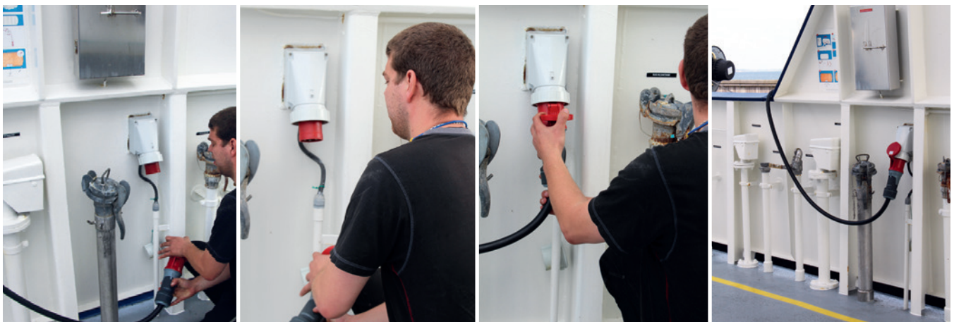
Staff connect to the shore power supply to commence charging the battery bank.
