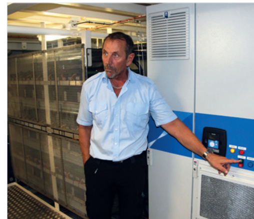
Søren Adersen explains the power conversion system which uses a VACON® NXC Air Cooled microgrid converter. The battery bank is on the left.
