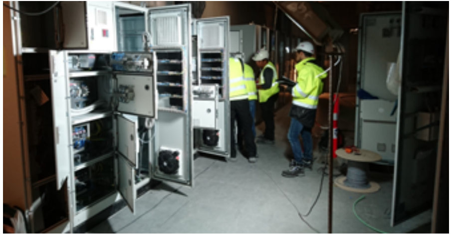
Panels from the station named "FBA" already placed on the technical floor and photographed during the tests carried out jointly by Systemair and H.S. Progetti.
