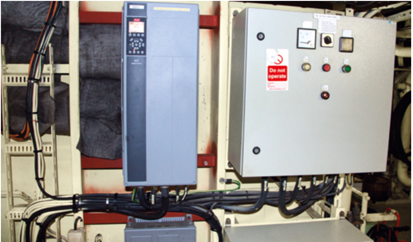
The sea water cooling pumps and engine room ventilation systems onboard the vessel are powered by Danfoss drives.
