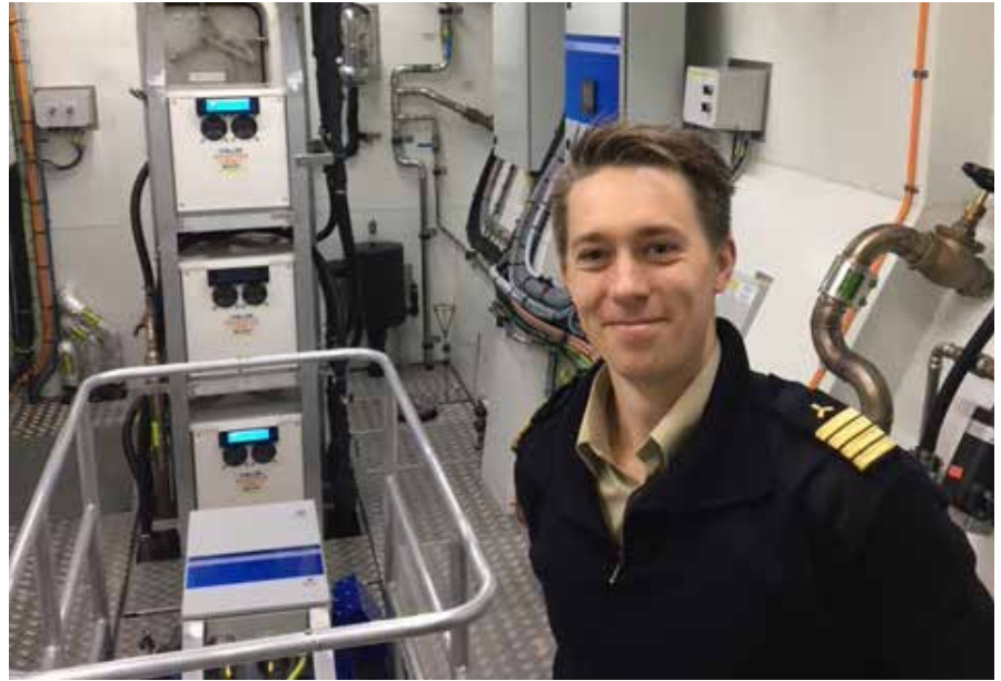
Lars Haugnes is highly satisfied with the performance of Danfoss drives and instrumentation installed in the machine room of Future of the Fjords , contributing significantly to protecting the pristine fjord environment.
