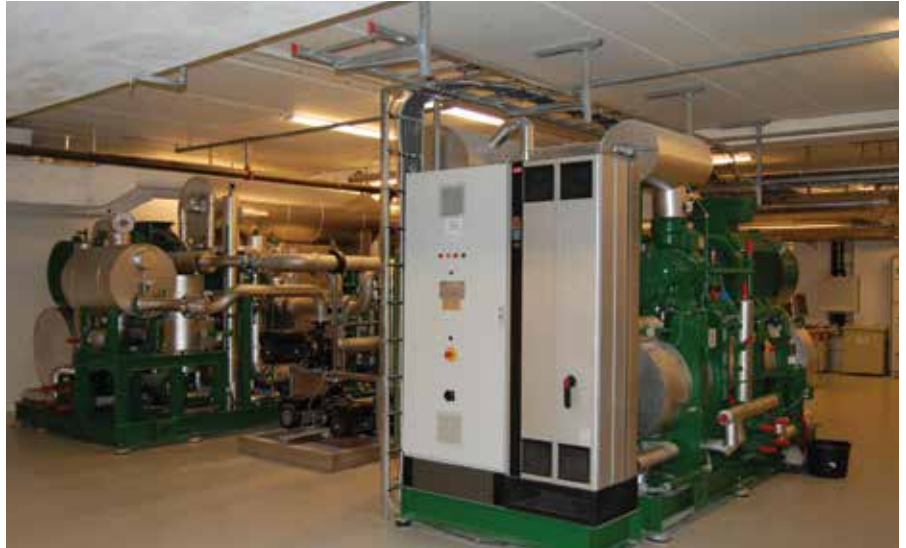
Two AC drives in the form of 355 kW VLT® HVAC Drive FC 102 IP54 control the screw compressors which enable the two GEA Greenco heat pumps with a combined performance of 2,400 kW to adjust the heat capacity continuously from low to full performance, with the same efficiency.
