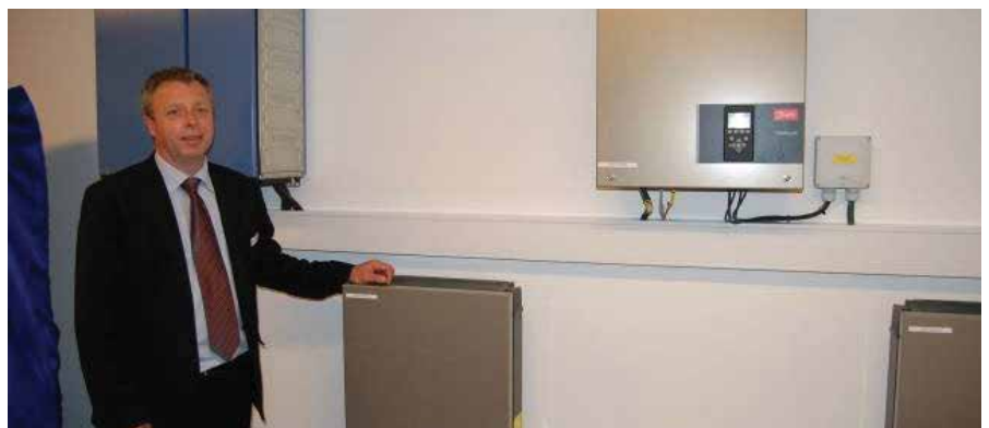
Peter Andersen, Copenhagen Towers' Property Director with Danfoss TripleLynx solar inverters
