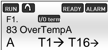
Figure 7.1-2, High temperature alarm on the NXP panel
