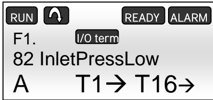
Figure 7.1-4, Low pressure alarm on the NXP panel
