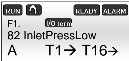
Figure 7.1-4, Low pressure alarm on the NXP panel
