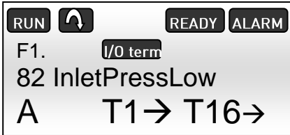
Figure 7.1-4, Low pressure alarm on the NXP panel
