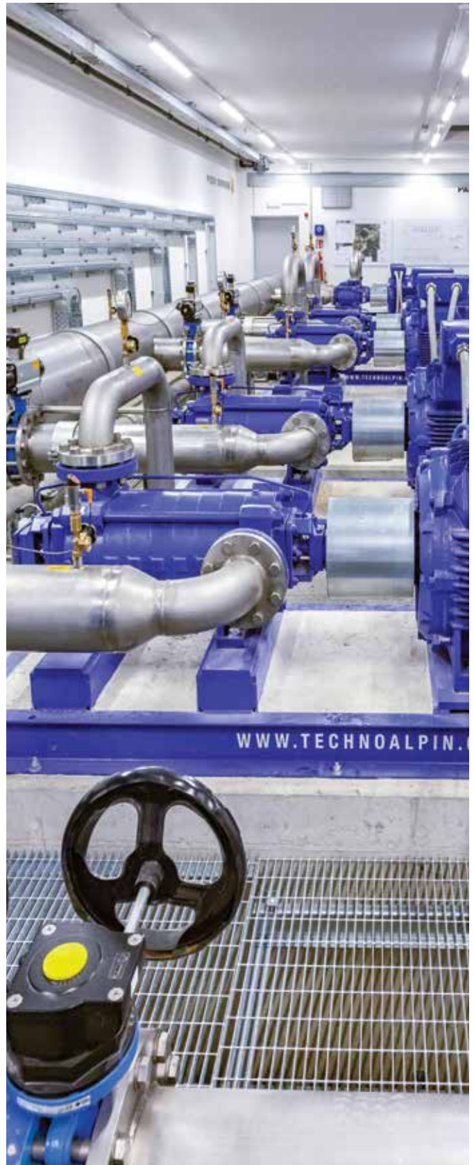
View of the main pumping station, located downstream of the plant.
